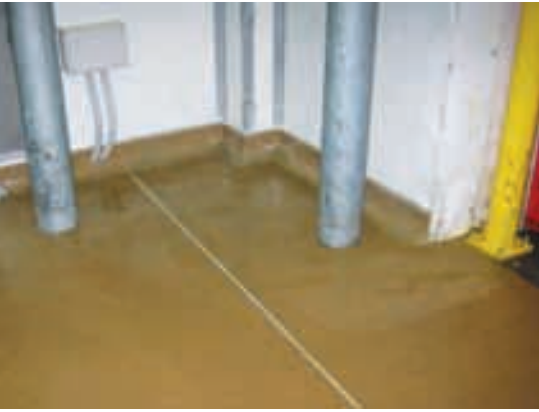
Aluminium coving was removed and replaced using very smooth Sika floor coving
