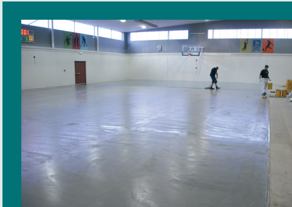
A 2mm base layer is applied on top of a 7mm shock absorbing mat.
