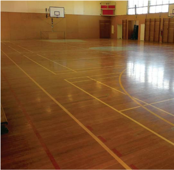
Before Pulastic Sports Flooring was installed
